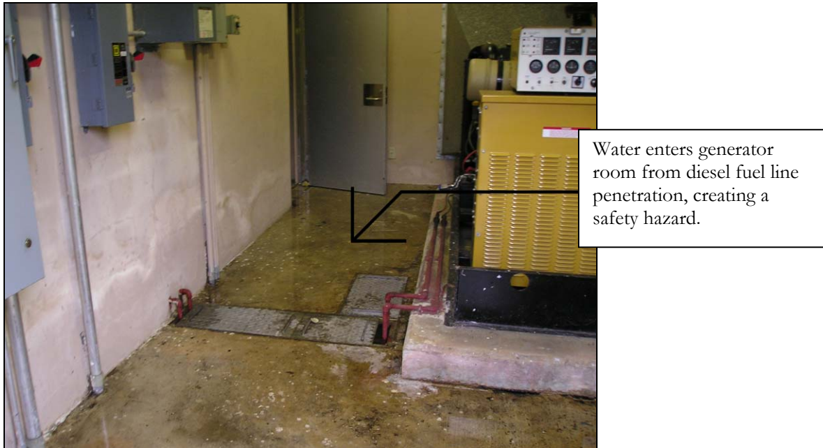
Figure 12-14 – Generator Room Fuel Line Penetration – Station A-3
