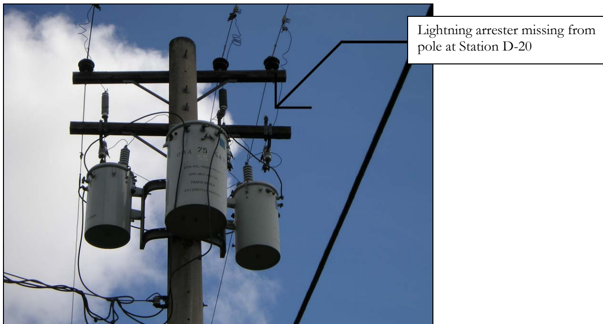
Figure 12-15 – Missing Lightning Arrester
