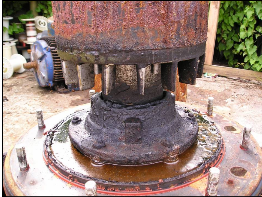
Figure 12-17 – Mechanical Failure in Submersible Motor
